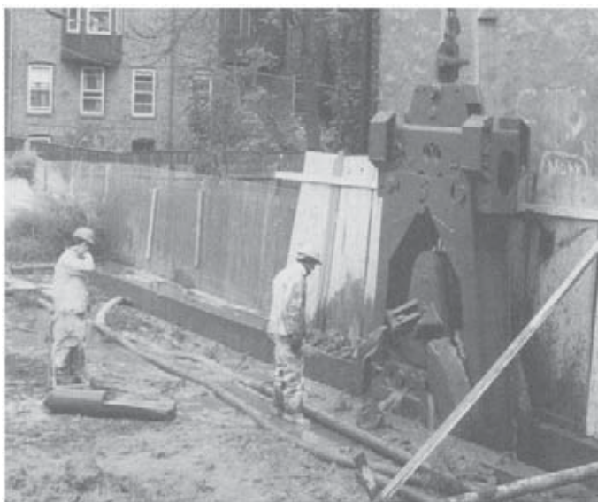
Fig. 23. One aspect of the process of participation in Boston’s Southwest Corridor project successfully involved abutting neighborhood groups in a review of approaches to construction of the tunnel. The consultation resulted in a decision to use a slurry wall system.
